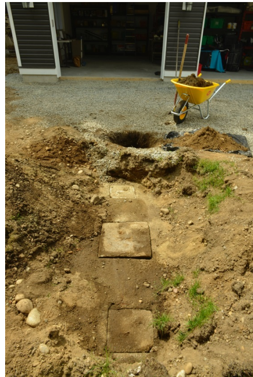
Septic lids exposed
