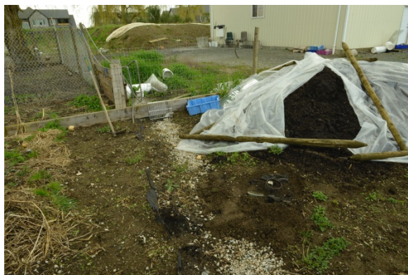
Drainage ditch installed along mound to divert to illegal pipe
